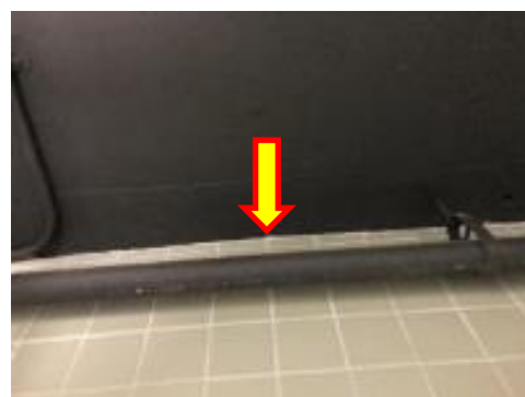
Photo 2: Uninsulated pipe – Men's Washroom.
