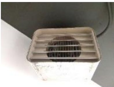
Photo 5: Electrical space heater – Women's Washroom.
