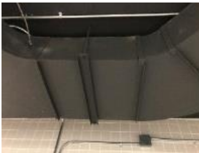
Photo 4: Uninsulated duct – Women's Washroom.
