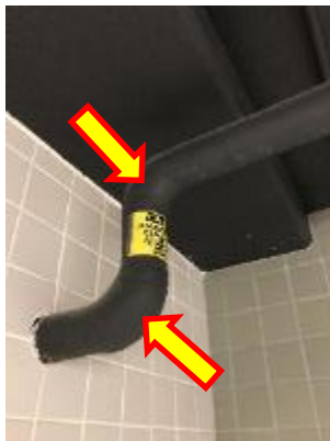
Photo 1: Asbestos-containing parging cement insulation on pipe elbows – Men's Washroom.
